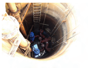
New Dry-Pit Submersible pumps in south collector well
