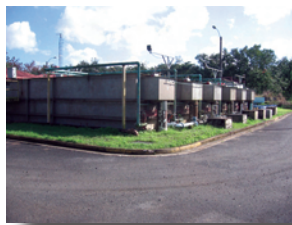
Plant sedimentation units
