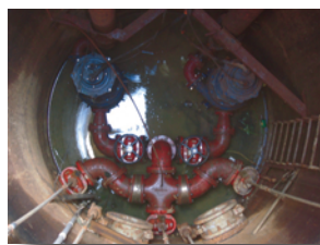
Pump suction manifold
