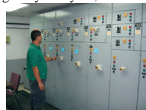
Plant operator at work with the new pump system
